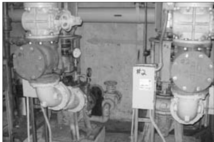
The two pumps, running simultaneously Thursday, August 11, caused sewage effluent to leak from an air release manhole along the line being taken from the Wastewater Treatment Plant to the Biddle Point Pumping Station and then out to Lake Huron.
