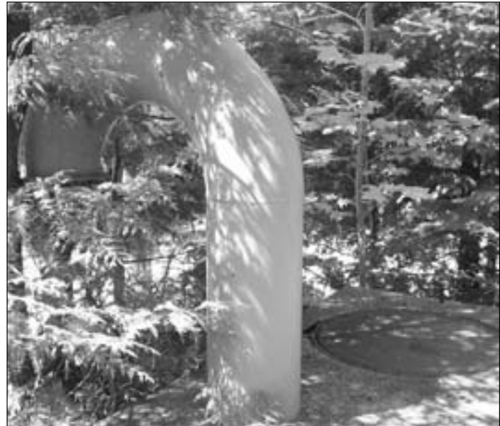
One of the air release manholes located on the line, which had leakage issues Thursday, August 11.
