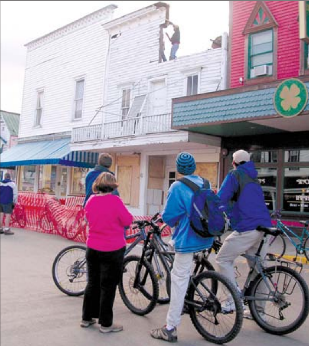
Bunker Construction began pre-demolition work on a collapsing Mackinac Island downtown building Wednesday, September 20. Demolition work was handled by Belonga Plumbing and Heating of St. Ignace and began the following day.
