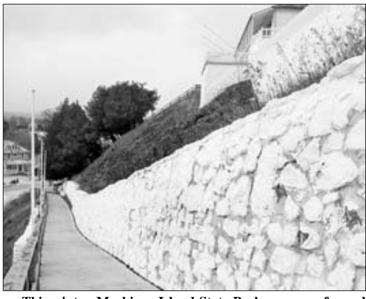
This winter, Mackinac Island State Park crews performed some patch work on the 226-year-old limestone walls at Fort Mackinac. The focus of a 2001 major restoration project, the walls are prematurely deteriorating, say park staff.
