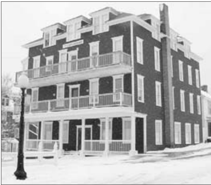
Deteriorating and no longer used, the brick chimney on the Windsor Hotel is slated for removal. The Mackinac Island structure is owned by Grand Hotel and used for employee housing.
