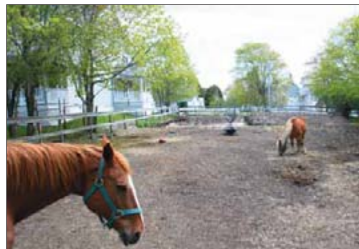
Horses meander about their corral Monday, May 21, ignoring foundation work that has begun on the property. Ground preparation for one of the homes can be seen near Mission Street. Three condominium housing units are planned for the lot.
