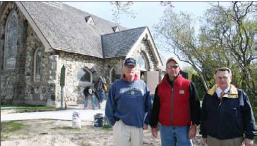
The outside remodeling work at Little Stone Church will be completed this week, said Pastor Vincent Carroll (left). Checking out the progress of the job, Monday, May 21 are Randy Stuck (center), building and maintenance manager for the church, and Buzz Waggoner, congregation president. The work was performed by Winberg Masonry Incorporated of St. Ignace. Winberg crew in the background are (left) Eric Engle, Aaron Winberg, and Matt Matson.
